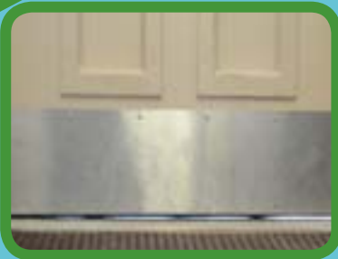
Above: Unsealed doorway provides pests with direct entry to the building.
