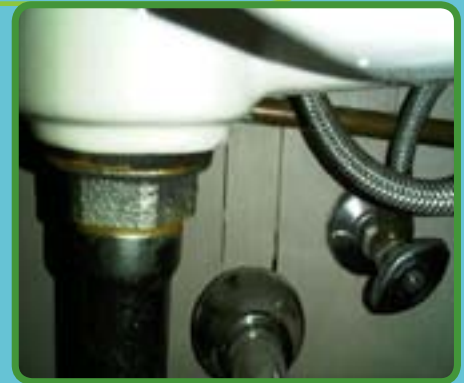
Above: Sealed pipes under sink.
