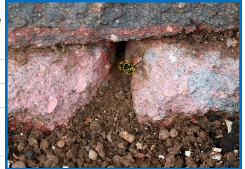
Western yellowjacket nest entrance at the base of a brick wall. W. Cranshaw
