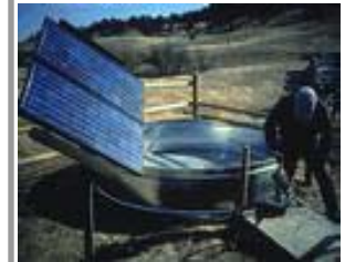
Solar Panel and Tank
