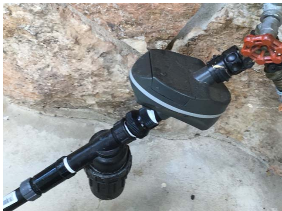
Fig. 27. Timer Controlling the Drip System Connected Directly to the Outdoor Hose Connection for City Water. Directly Below the Timer is Back Flow Prevention Valve, Followed by Filter and Pressure Compensator to Reduce City Water Pressure to Level Suitable for the Drip System.
