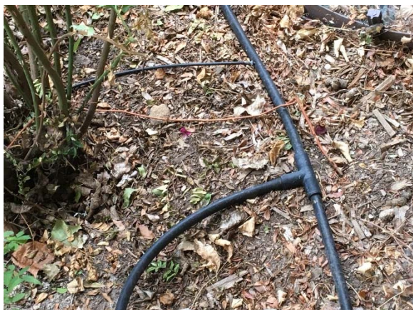
Fig. 28. Main 2 cm Drip Line With T Junction to Another Section Plus Capillary Line Going to Individual Roses.
