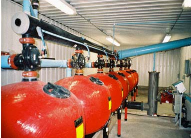
Fig. 21. Bank of Sand Filters Used in Large (20 ha) Commercial Drip Operation to Make Certain no Particulate Material will Plug Emitters
