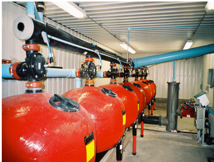
Fig. 23. Bank of sand filters for filtering water for commercial large scale drip system, even when using well water with limited suspended particulate material.
