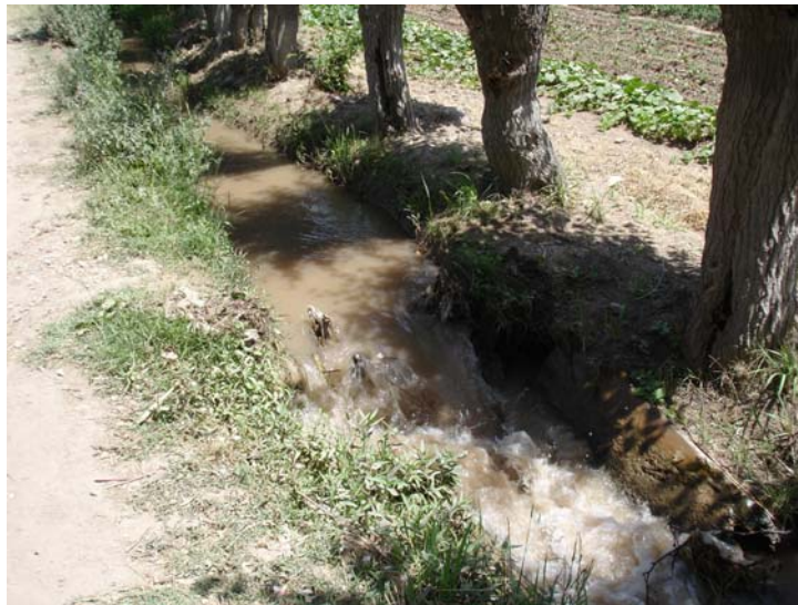
Fig. 10. Improvised check/drop structure made of some riprap used to attempt to control canal water.
