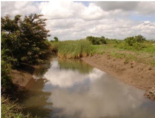
Fig. 21. Main canal with weed growing across sections of the canal and reducing flow.
