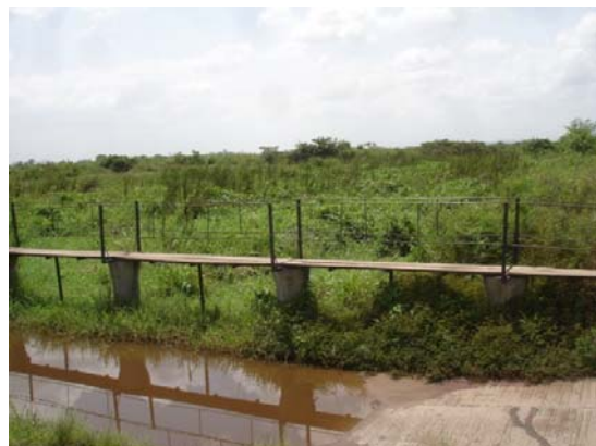
Fig. 22. A ford in the drain with footbridge and behind the drain fully blocked with weeds.
