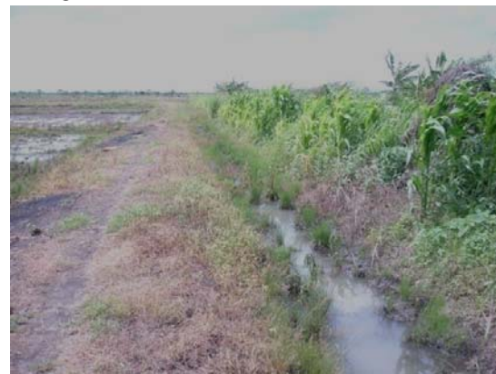
Fig. 25. Typical tertiary canal in need of cleaning but not in vested interest of those designated as responsible for cleaning.
